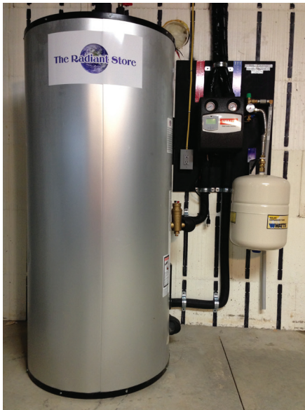
Water heated by the sun's energy is stored in a storage tank.
